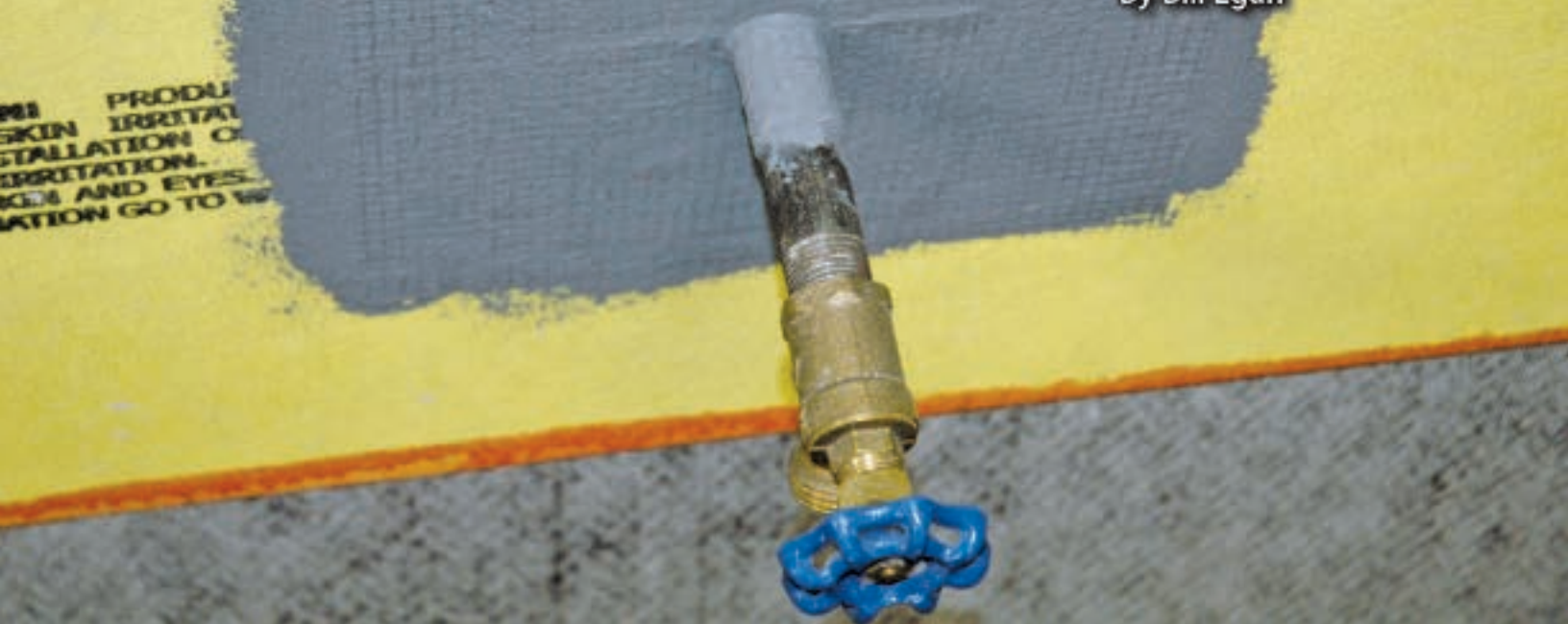
Figure 1. An example of a penetration that has been made air- and watertight using a reinforcing mesh/fluid-applied material.
