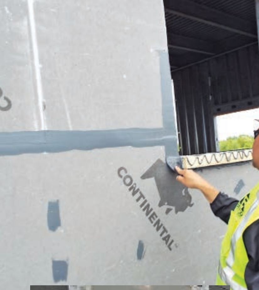
Figure 2. An accessory used to transition between joints of adjacent pieces of sheathing is visible in this photo.
